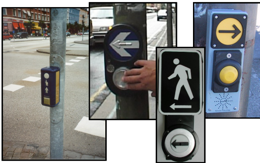
APS & Pedestrian Pushbuttons— R307 & R209.1 109
